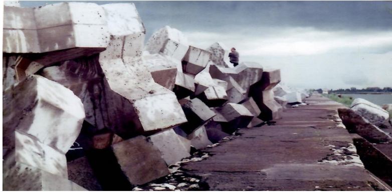
Fig. 4. Tetrablocks in Poti Port, Georgia, [11]
