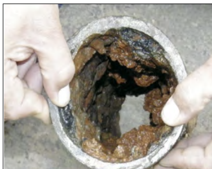
Fot. 1. Rura żeliwna Ø100mm z osadami (bud. 1939 r.) Pic. 1. Cast iron pipe Ø100mm with deposits (building 1939)
